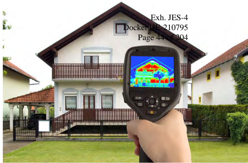
A home's insulation and drafty spots viewed through an infrared camera. Image source: https://www.energy.gov/energysaver/thermographic-inspections
