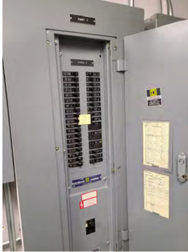
Existing age of Panelboards in Building
