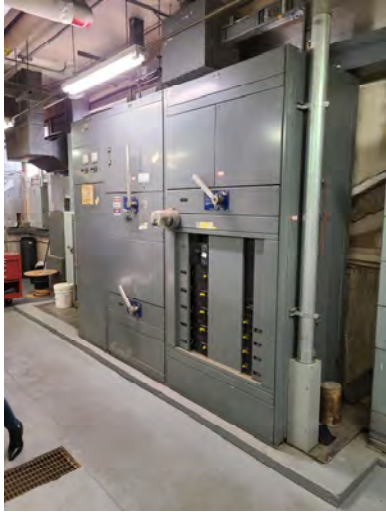
Existing Main 480/277V 3,000 A Switchboard
