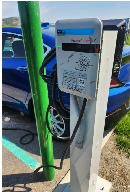
Figure 17: Station hit by vehicle identified during an inspection.
