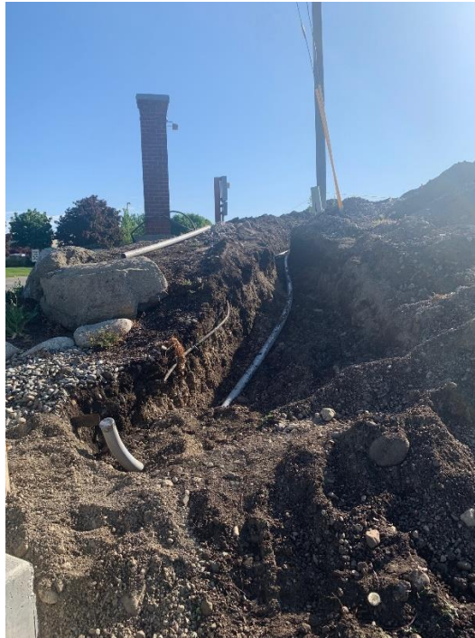
Figure 14: Conduit – Trailhead Golf Course
