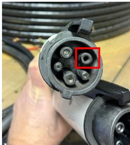
Figure 18: Connector pin damaged (missing internal piece) after utilization of a non-Tesla adapter.
