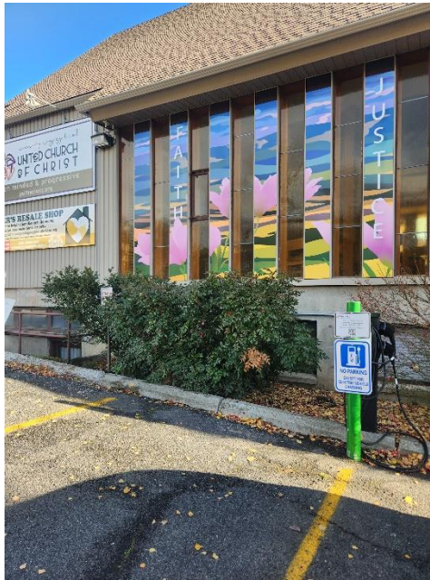
Figure 8: Public charging installation
