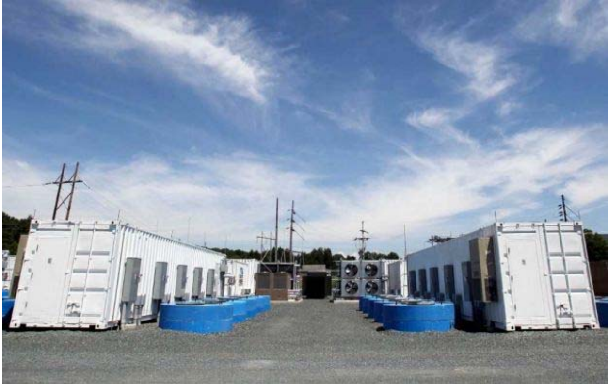
Figure 24- Flywheel Plant New York
