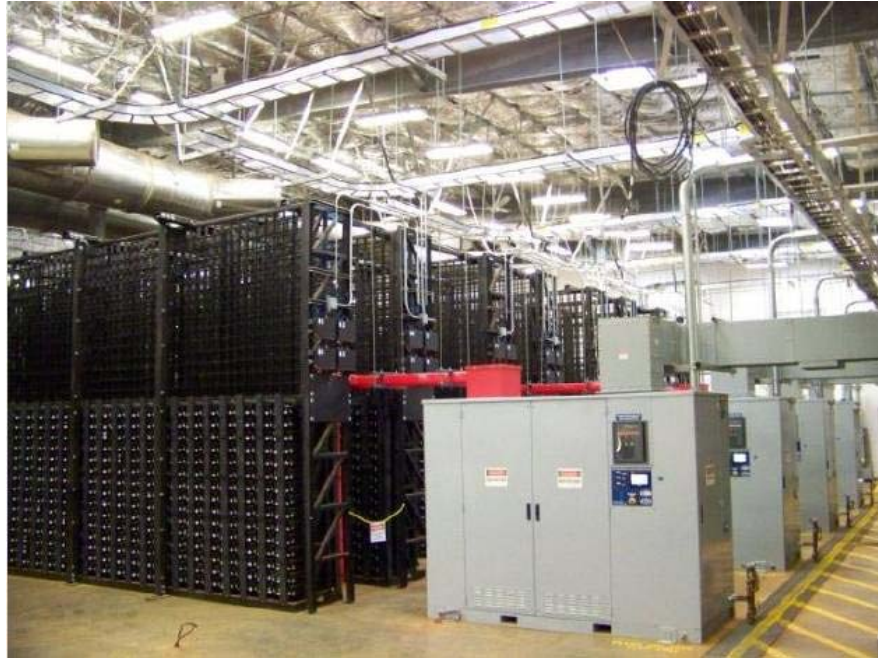
Figure 15- PowerCell™ Stacks with PCS
