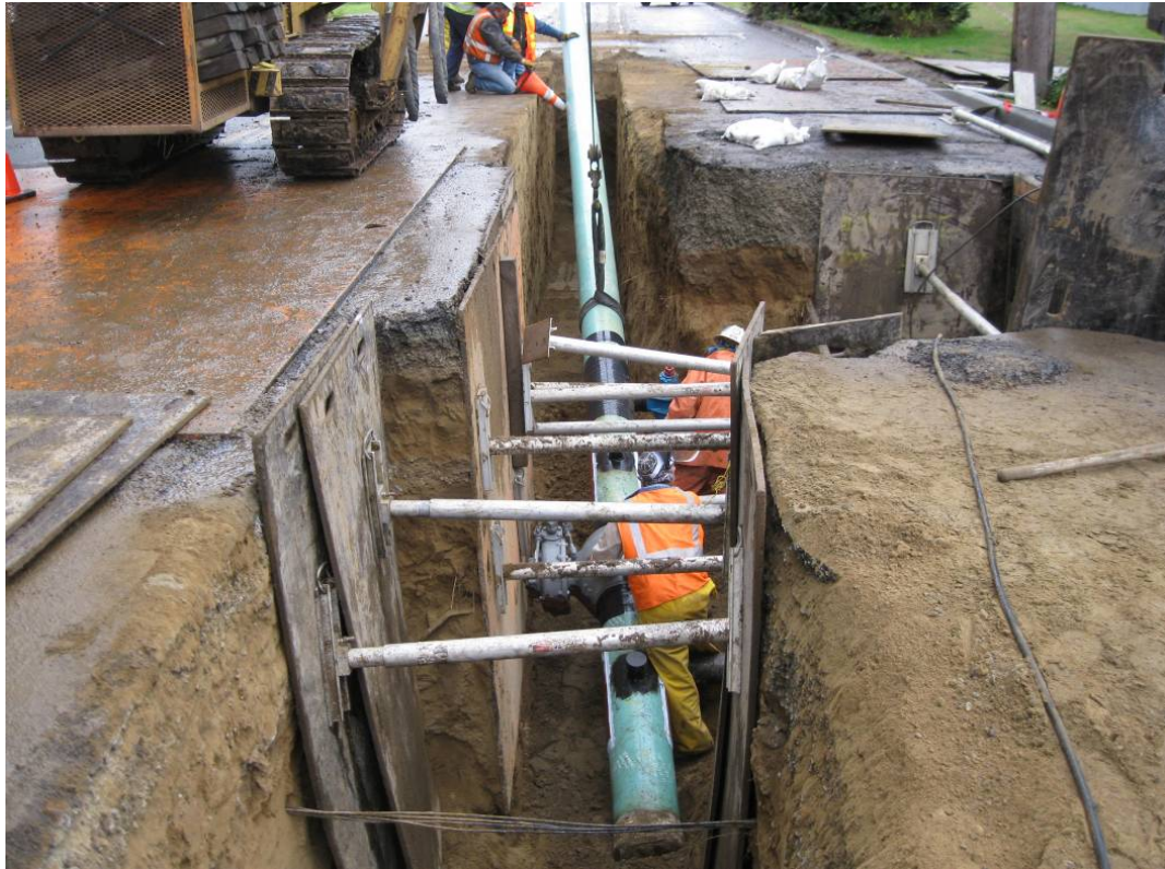
Figure 3-6: Lacey-Fones Road, 12-Inch Diameter Supply Pipeline, In-Service 2009
