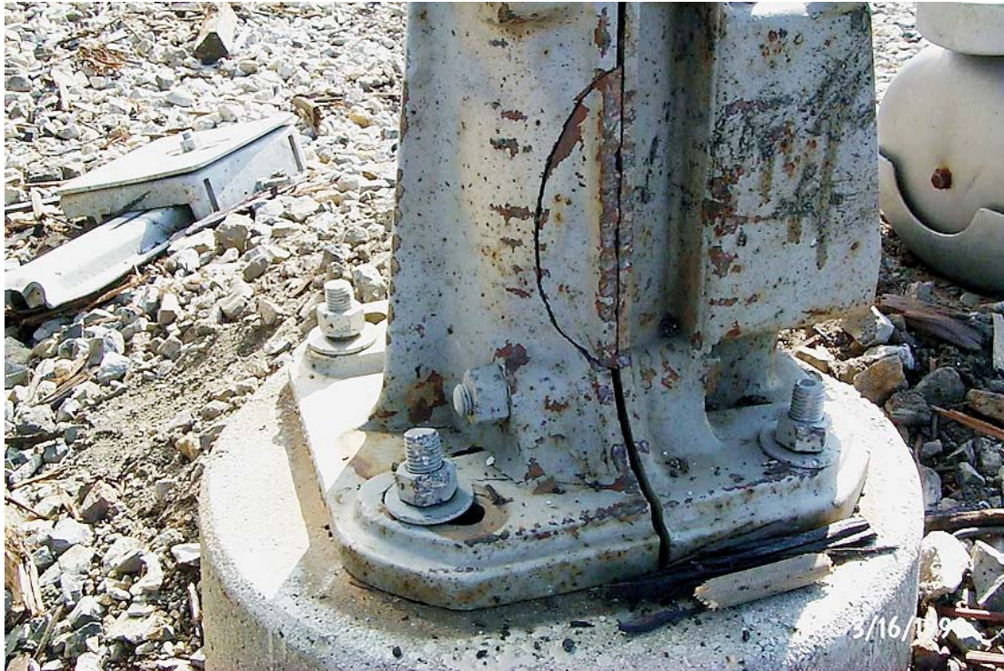
Figure 7. Cracked cast metal base of the west-side crossing gate.
