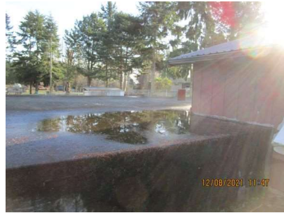
Large Storage Tank - Ponding
