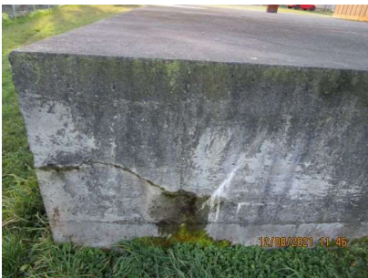
North Side Large Storage Tank
