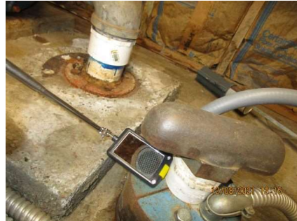
Small Storage Tank Vent
