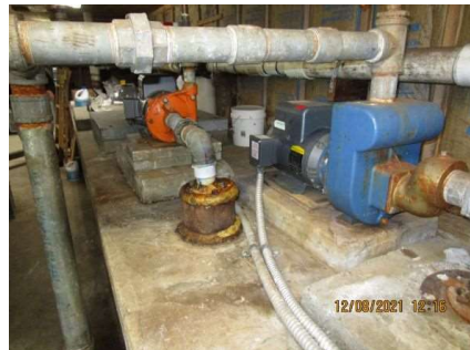
Booster Pumps for Small Storage Tank
