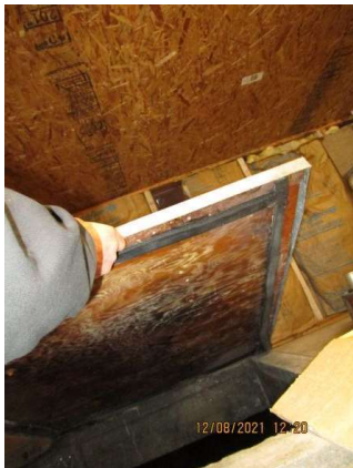
Small Storage Tank Hatch Gasket
