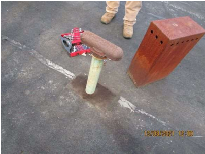
Large Storage Tank Vent
