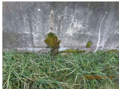
North Side Large Storage Tank
