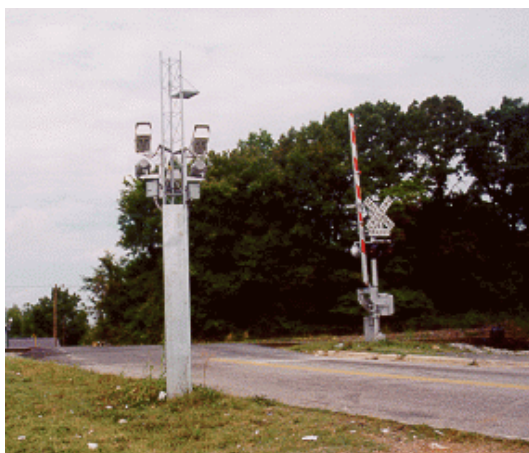
Figure 5. Photo Surveillance Hardware
