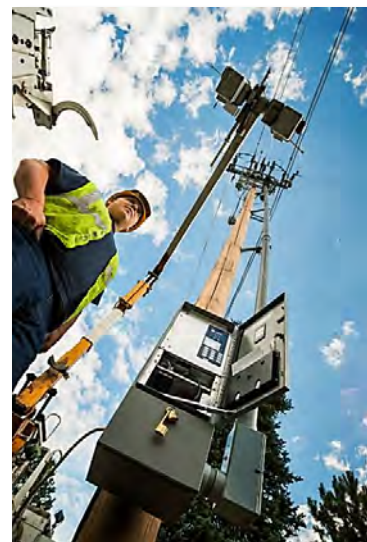
Adding Grid Modernization Technology to a Feeder
