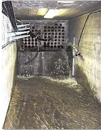
Flooding in the Downtown Network underground system after a rainstorm
