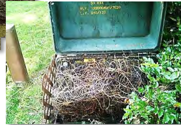
Below: Vines Growing Inside a Transformer Box
