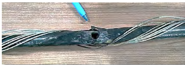
Old cable, susceptible to failure
