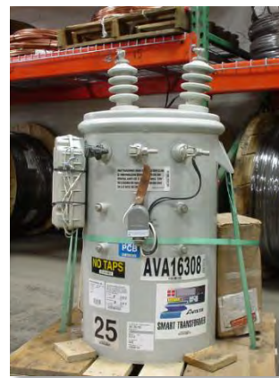
Left: "Smart" transformers provide the exact amount of power needed, respond to fluctuations and act as a voltage regulator
