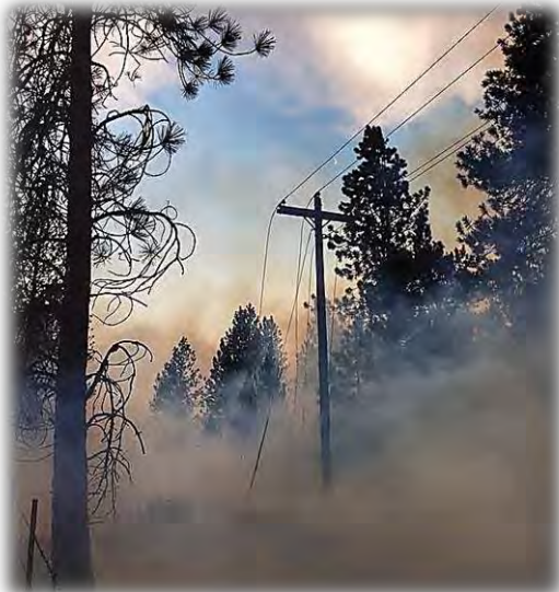
Distribution Line destroyed by wildfire
