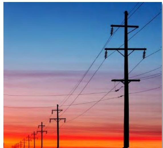
Transmission Poles showing distribution lines “underbuilt” below the transmission lines, which puts additional strain and wear on the poles
