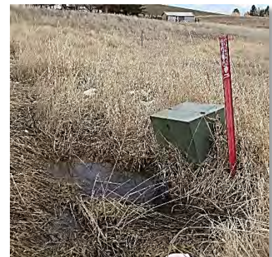
Underground equipment now in a bog
