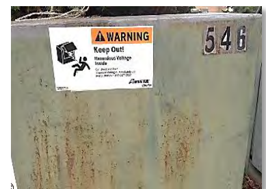
Below: Paint failure can lead to rust-through of cover
