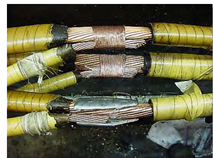
Downtown network crew beginning the process of filling cable with lead to create a solid splice; this type of work is considered an art
