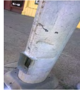
Figure 20: Rust, No Cover, Damage
