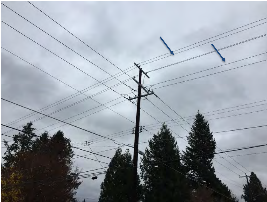
Figure 4. Paralleled 336 ACSR trunk at Cedar-Walnut & Wabash
