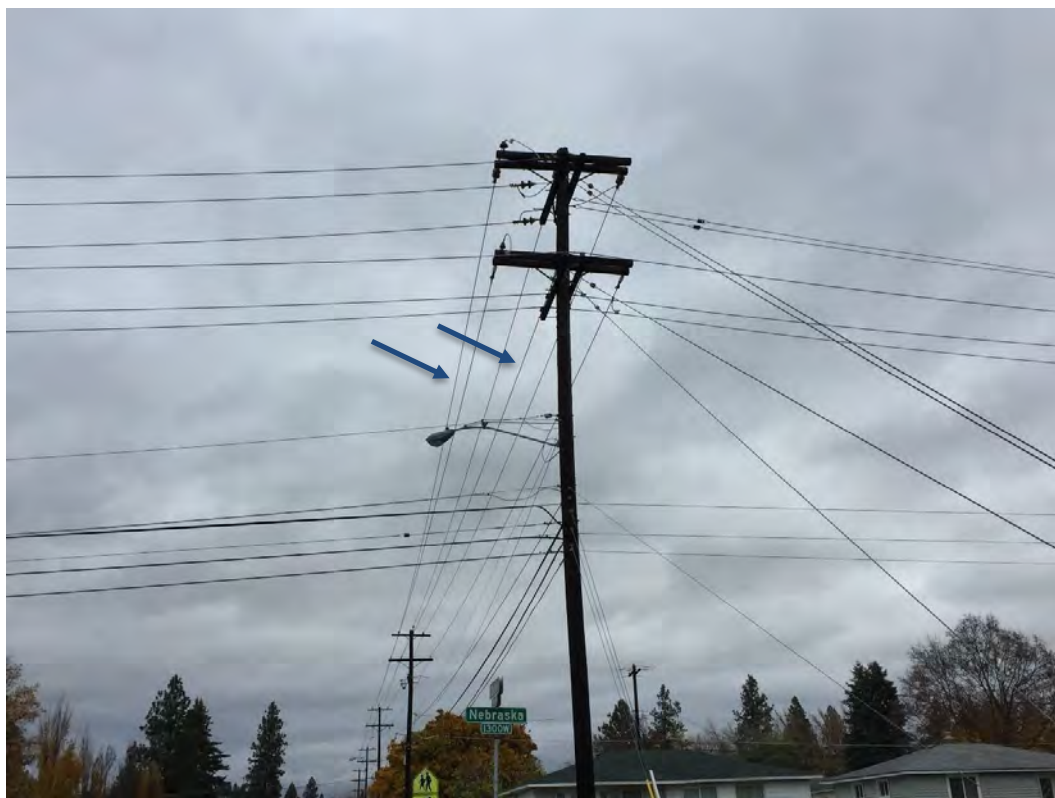
Figure 5. Paralleled 336 ACSR trunk at Cedar & Nebraska
