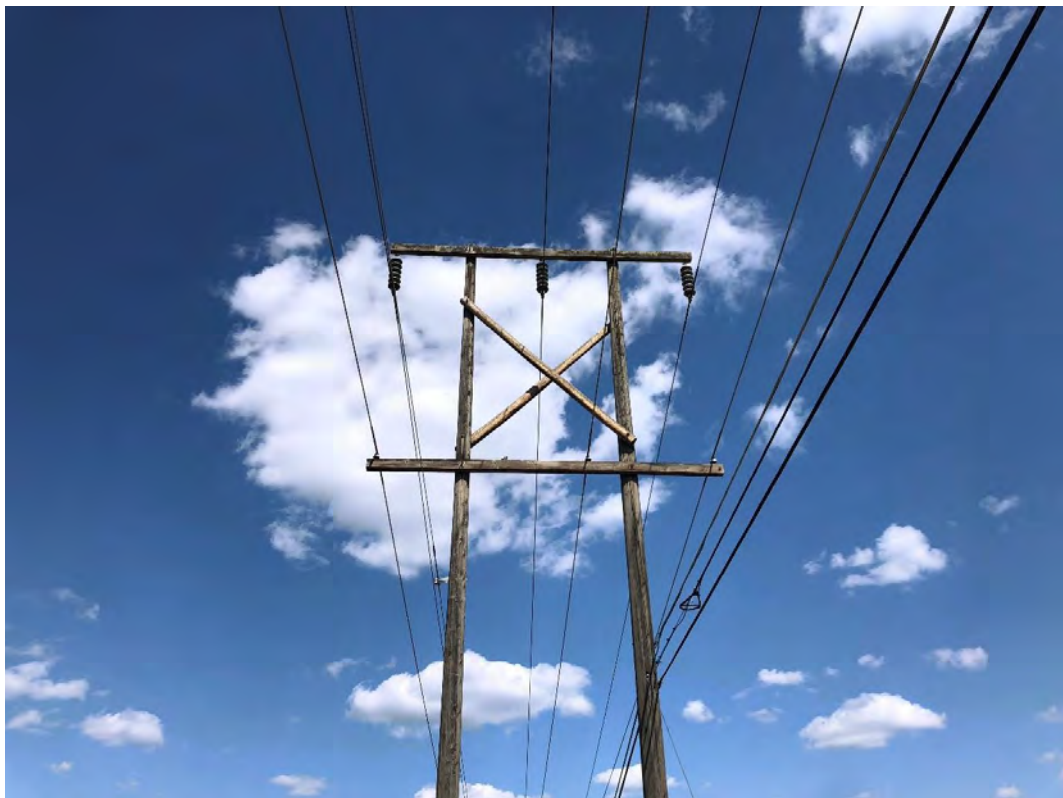
Figure 33. Three-Phase Primary River Cross at Pole #000053
