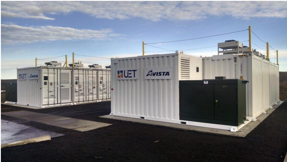
Turner Energy Storage Project, Pullman, WA
