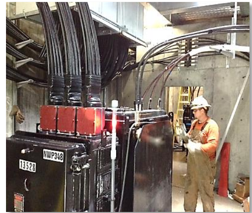
Downtown Network Vault
