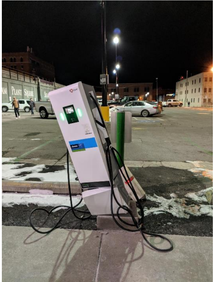
Figure 31. EVSE damage from a vehicle impact
