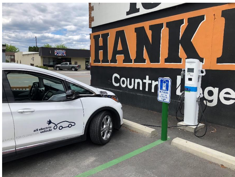
Figure 15: Public EVSE installation in partnership with the City of Colville
