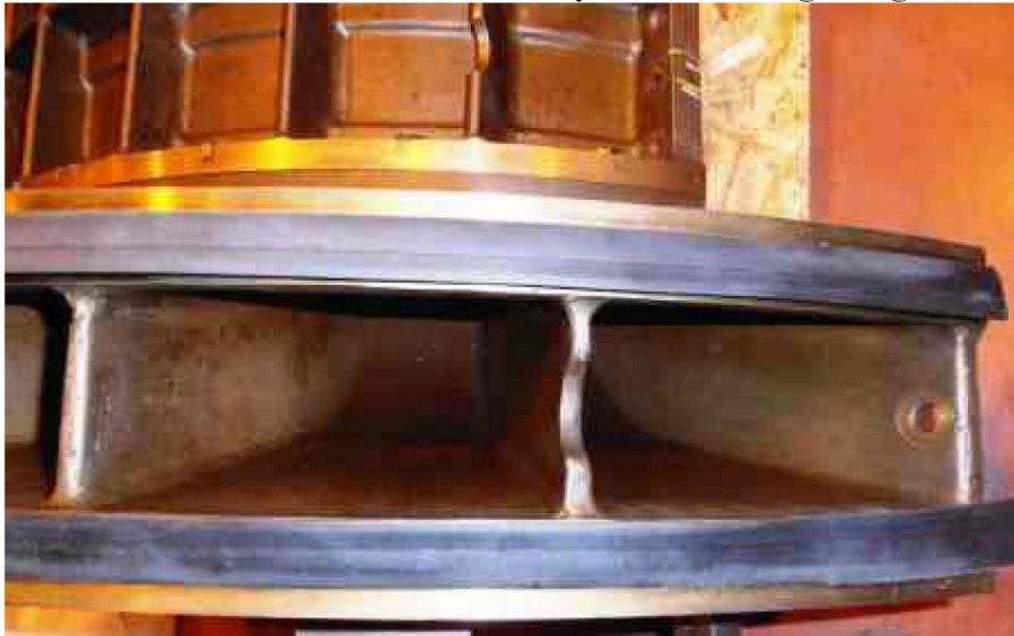
5 RS Generator Blower Stationary Blade Casting Gouges
