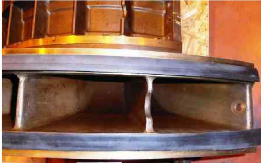
RS Generator Blower Stationary Blade Casting Gouges
