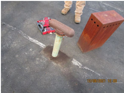
Large Storage Tank Vent
