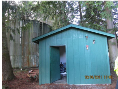
Storage Tank and BPS
