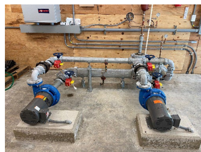
Booster Pumps in Transfer Station
