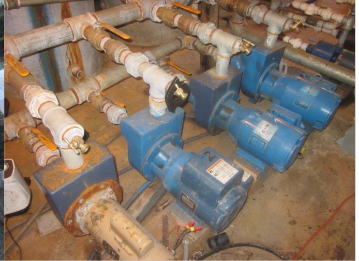
Lower zone booster pumps
