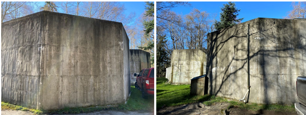
(L) & (R) Existing reservoirs – soon to be demolished once the new tank is finished and online
