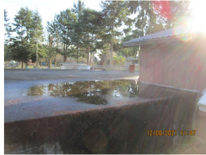
Large Storage Tank - Ponding
