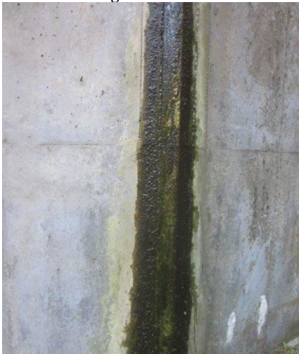
Leaking reservoir corner
