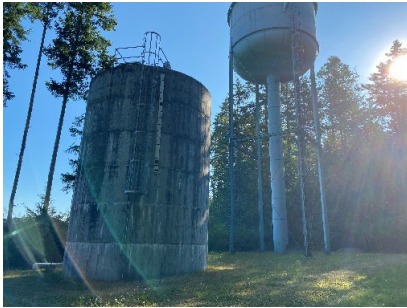
Tank 2 & 3 at Transfer Station
