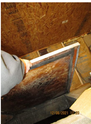
Small Storage Tank Hatch Gasket
