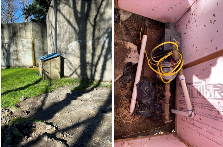
(L) Booster pump housing near reservoir (R) 1-HP Booster pump for 2 connections
