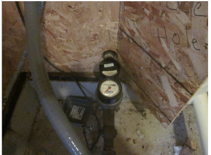
SO1 water meter
