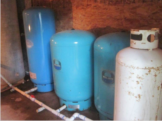
Upper zone pressure tank
