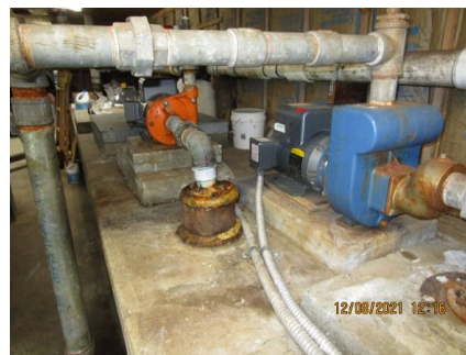
Booster Pumps for Small Storage Tank
