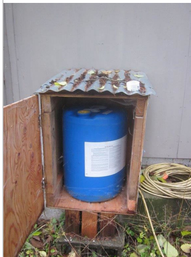
Chlorine solution storage
