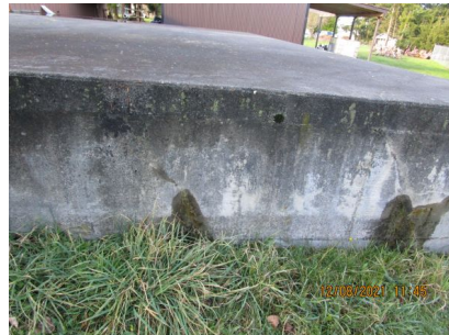
East Side Large Storage Tank
