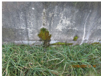
North Side Large Storage Tank
