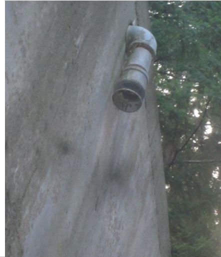
Water tank overflow
