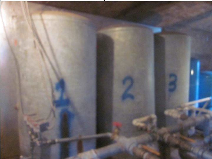
Lower zone pressure tanks
