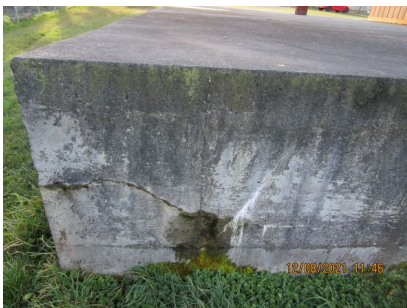
North Side Large Storage Tank
