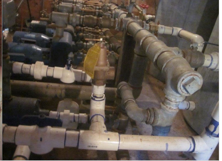
Pump house interior
