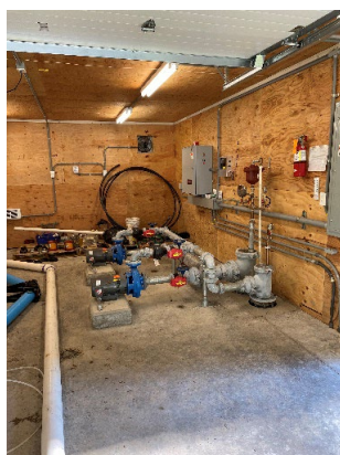
Booster Pump Transfer Station
