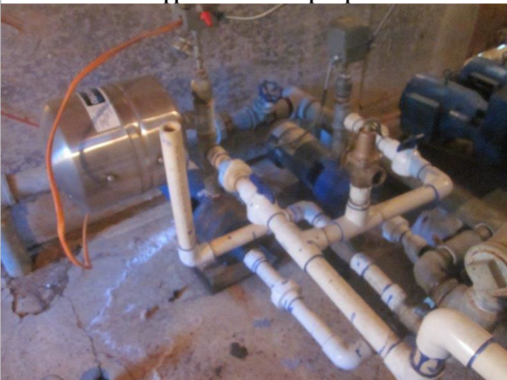
Upper zone booster pumps
