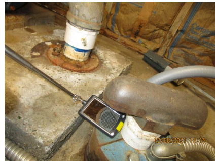
Small Storage Tank Vent
