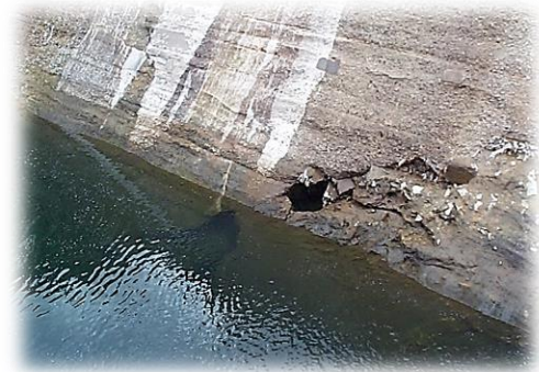
Long Lake Dam erosion
