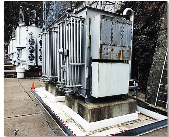
Cabinet Gorge Station Service
