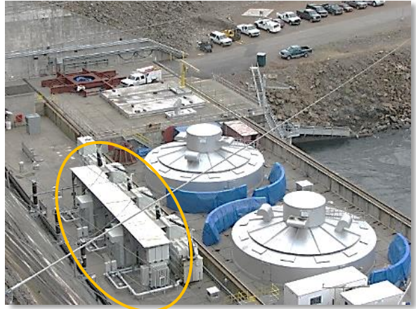
Noxon Rapids transformer bank
