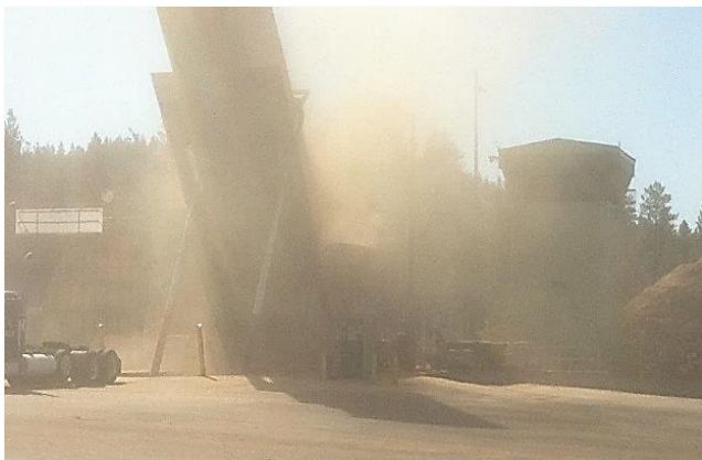
Dust created from dumping loads into undersized equipment, an environmental and air quality concern
