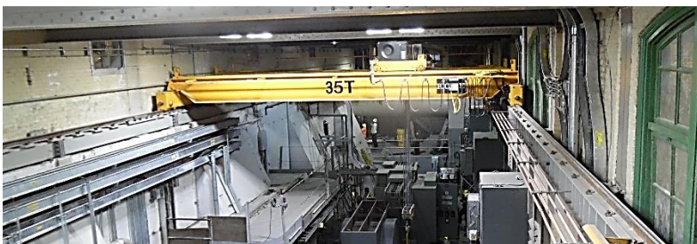
One of Nine Mile's two powerhouse cranes
