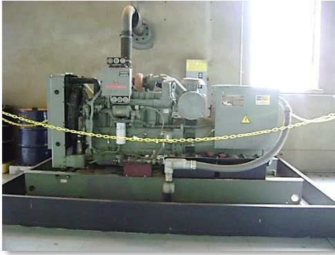
Current Long Lake emergency generator
