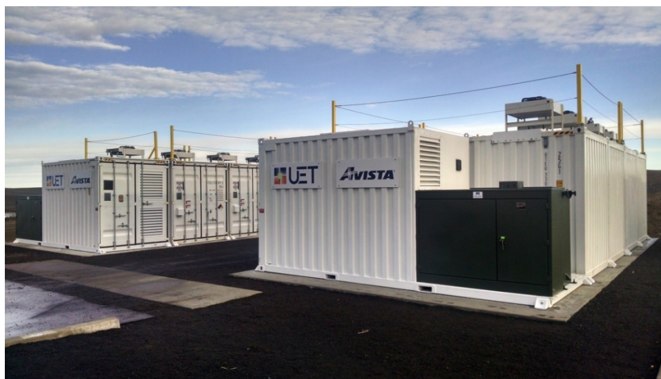
Turner Energy Storage Project, Pullman, WA
