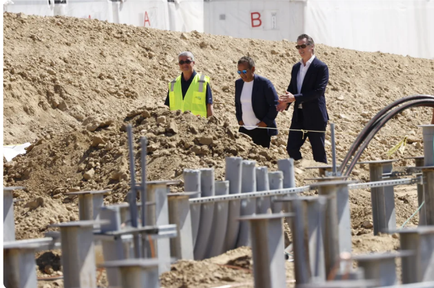
Jim Shandalov, vice president at NextEra Energy Resources, California Governor Gavin Newsom (R), and former Mayor of Los Angeles Antonio Villaraigosa (C) walk along the construction of the battery storage facility for a solar farm. (John G. Mabanglo-Pool/Getty Images) (Pool via Getty Images)
