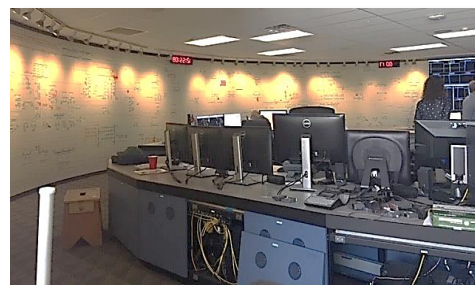
Above: One desk in System Dispatch: note the number of required screens and space needed
