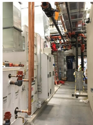
Facilities work involves complex systems like those above and on the left as well as historically significant assets such as the Steam Plant in Downtown Spokane (far left)
