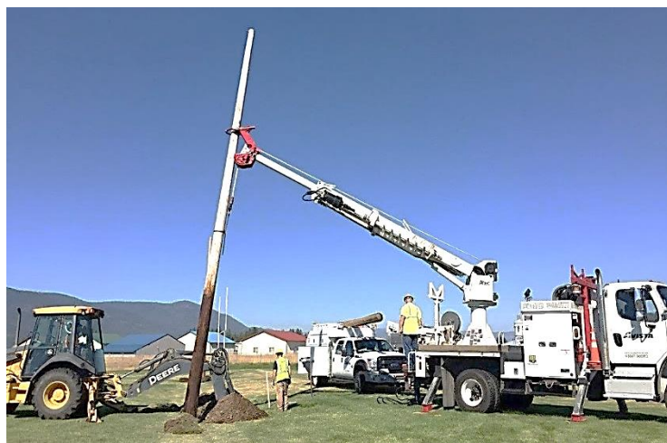
Specialized equipment needed to set a pole – a backhoe, a service truck, and a digger derrick.
