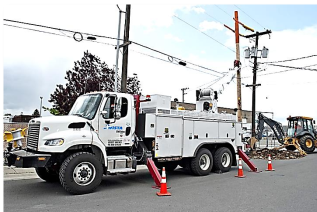
Safety cones are set up around Avista vehicles to protect the public
