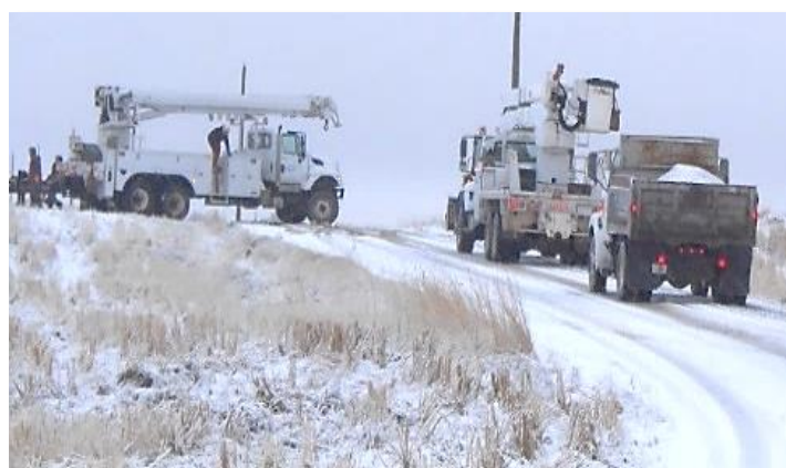
A variety of vehicles may be needed to handle an outage or perform a large installation or repair
