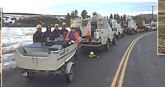
Crews must use a boat to access a pole that crosses a river.
