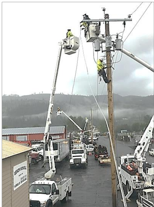
Using a variety of different sizes of bucket trucks and support vehicles to repair storm damage in Kamiah
