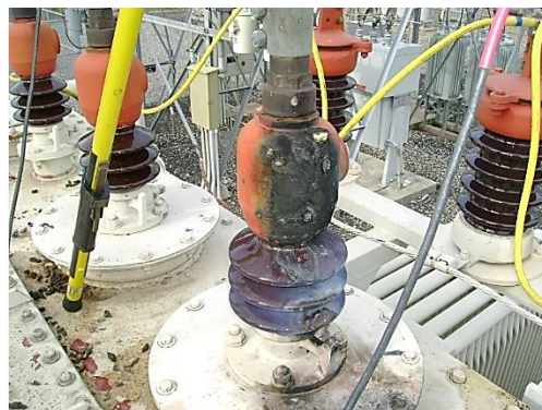
Animal-caused damage at Deer Park Substation
