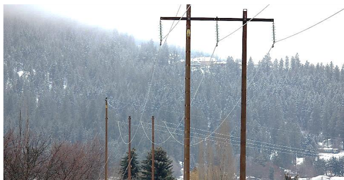
Ninth & Central transmission line
