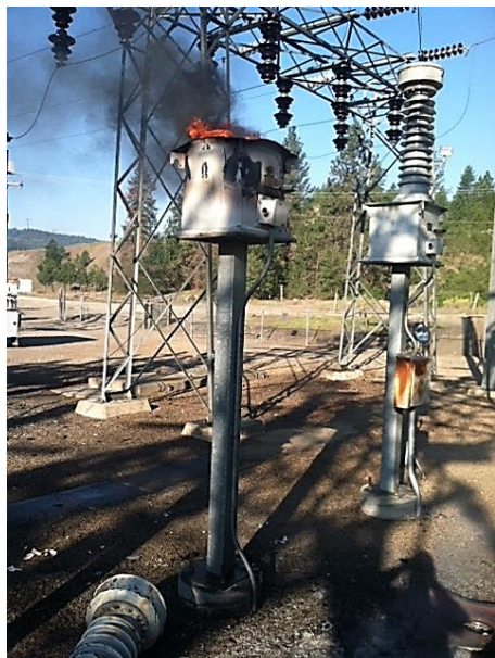
Switchyard equipment failure at Little Falls
