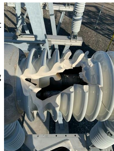
South Othello circuit switch interrupter failure
