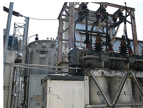
Cabinet Gorge 230 kV Substation breakers
