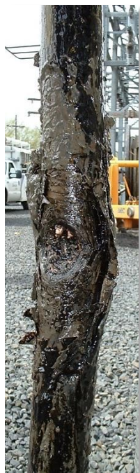
Failed cable at Moscow City Sub
