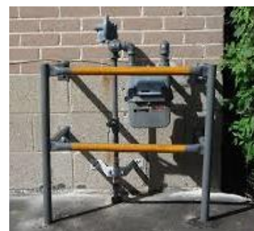
Gas Meter Barrier
