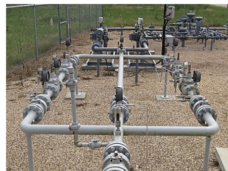
Natural Gas Regulator Station
