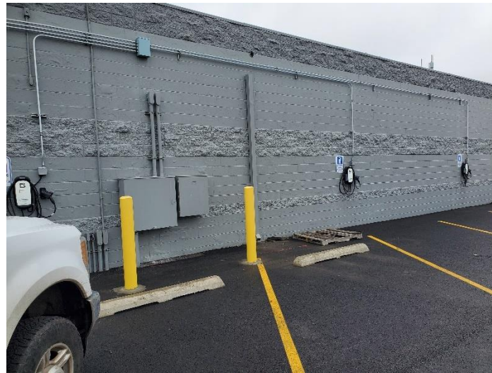
Figure 8: Fleet charging installation
