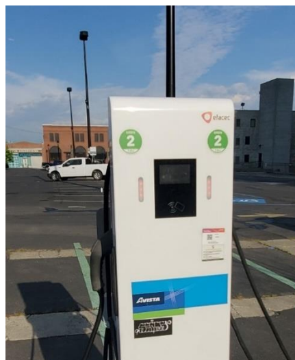
Figure 16: ACL2 station with both ports faulted (red indicator lights)
