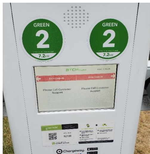
Figure 15: ACL2 station charging error code
