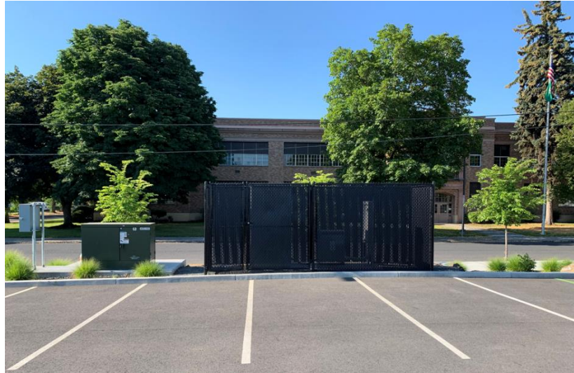
Figure 11: Fencing surrounding electric gear at The Hive – Spokane, WA (2022)
