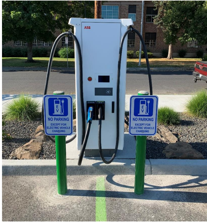
Figure 9: ABB Terra 184 DC Fast charger at The Hive – Spokane, WA (2022)
