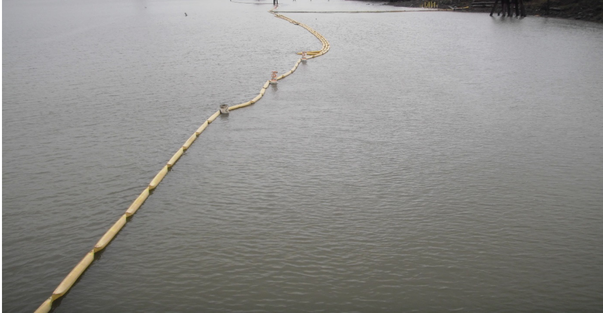
Photo 1 Centerline Oil Boom Placement from Dock to Dolphin with Three Mariner Warning Buoys at Pilot Cap Area (1/18/2023)
