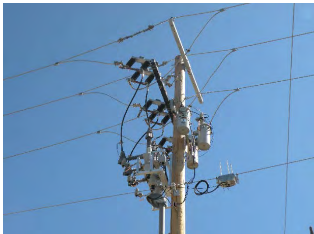
Distribution midline reclosers will play an important role in Avista Next Generation Dry Land Mode program. The ability to quickly detect and de-energize circuits is paramount to reducing fire ignition events.
