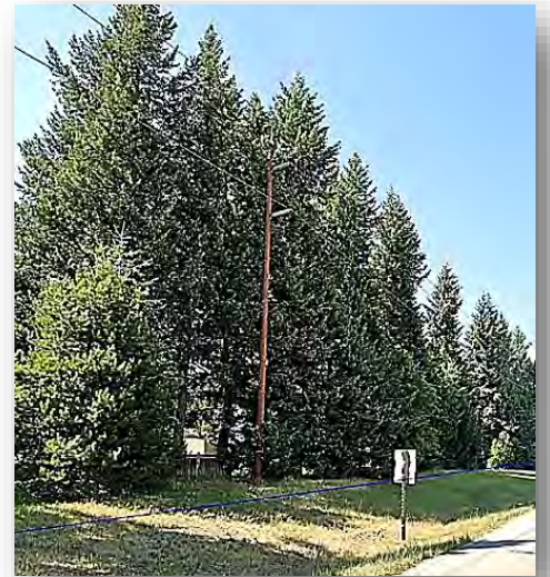
CDA-Rathdrum 115 kV along US Hwy 95
