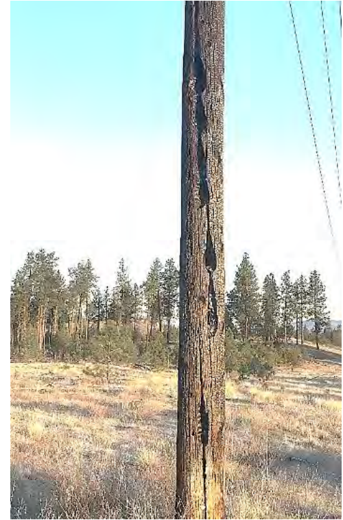
Pole fires generally occur on wood poles with wood crossarms. Since the early 2000's, Avista has adopted fiberglass crossarms as the standard unit. Replacing wood crossarms in elevated fire risk areas is a component of Wildfire Resiliency.
