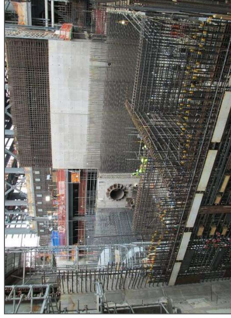
Unit 3 North Auxiliary Building
