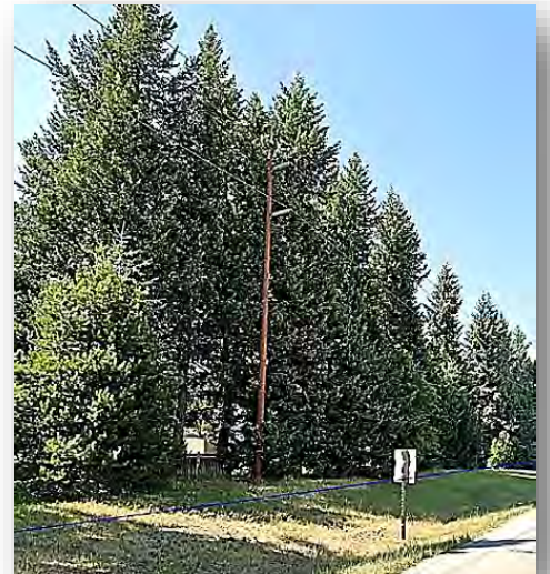
CDA-Rathdrum 115 kV along US Hwy 95
