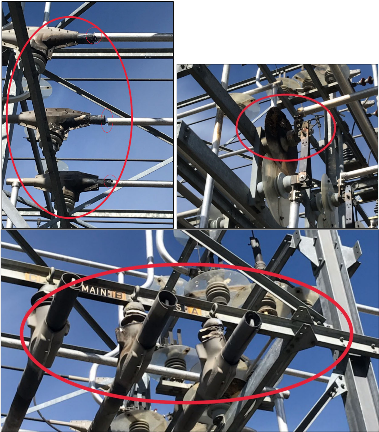
Figure 1: Photos of damaged equipment.
