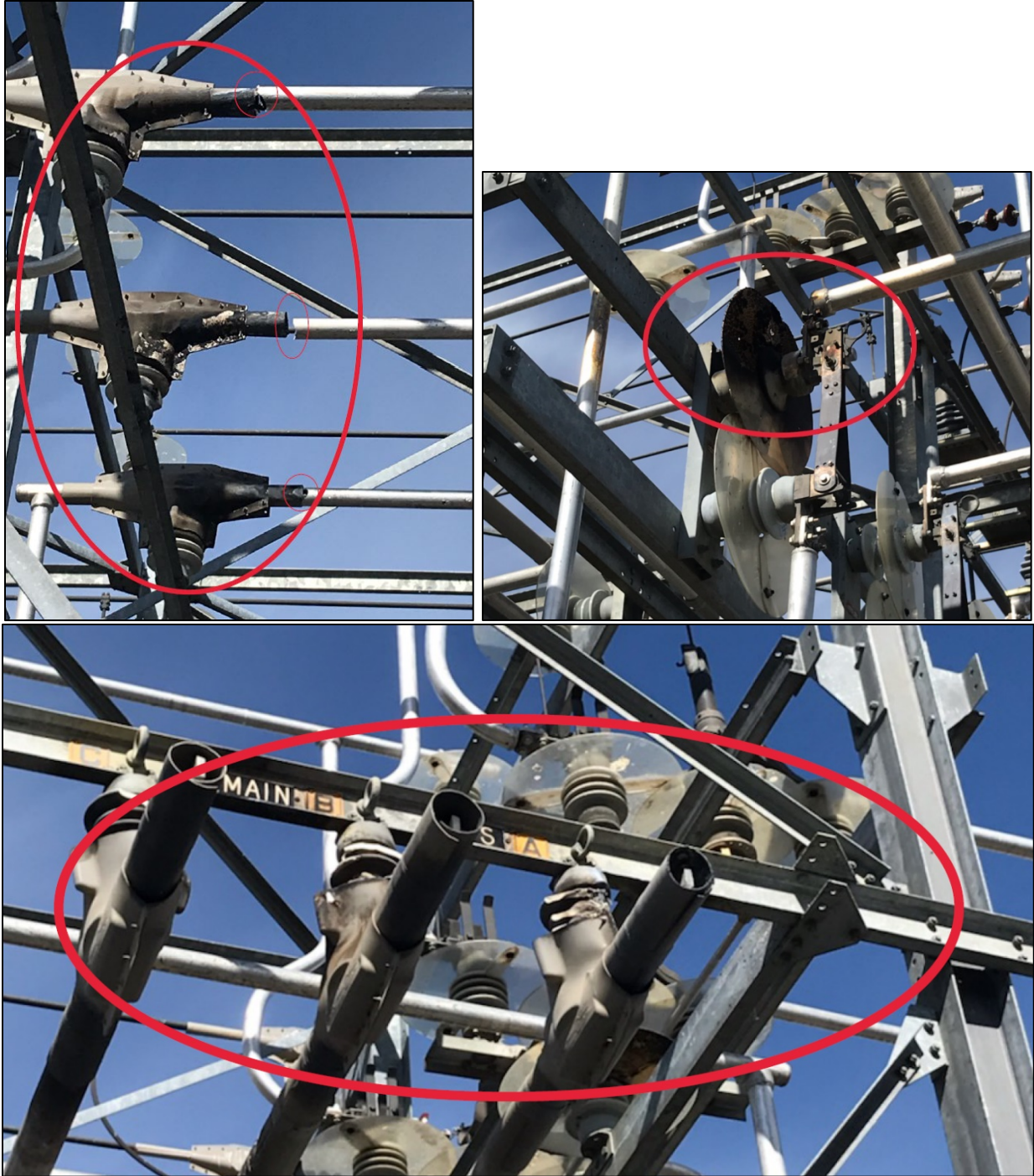
Figure 1: Photos of damaged equipment.
