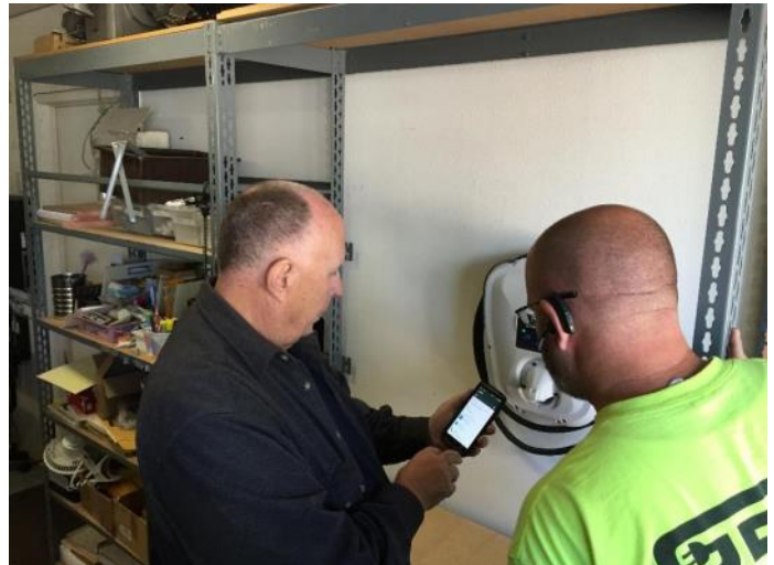
Residential EVSE installation with direct load management capability via homeowner WiFi and the Greenlots network (2017)
