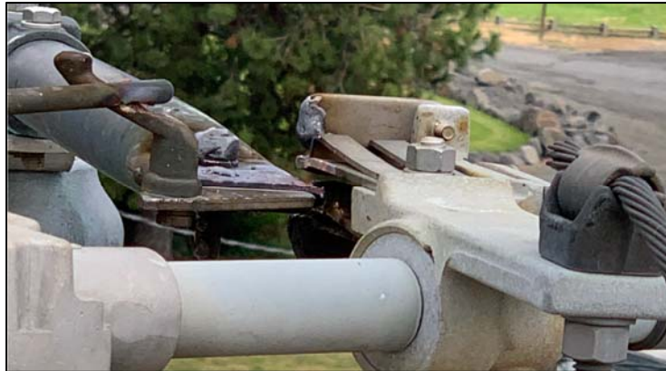
Figure 1. Damaged line switch
