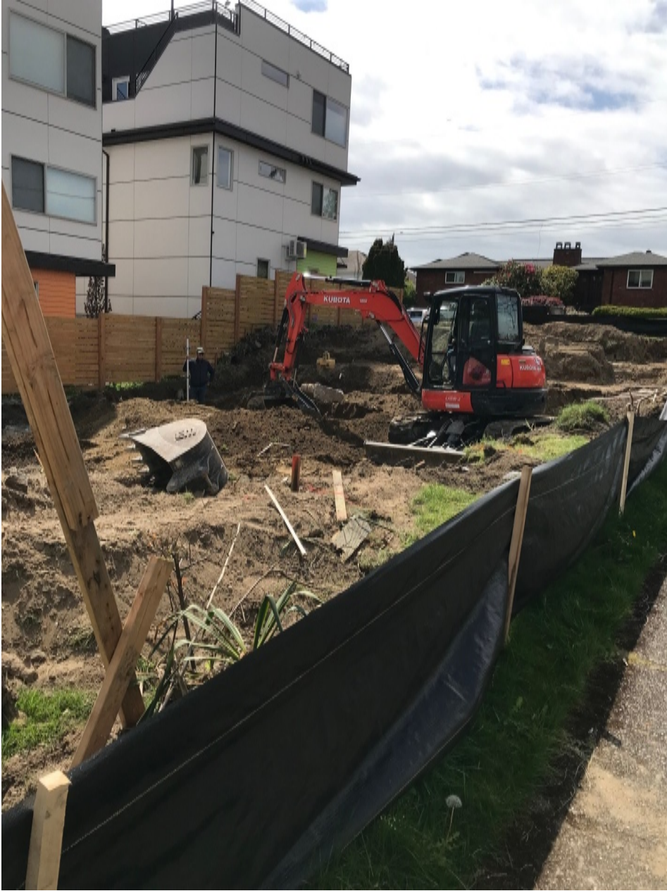
Pictures showing excavation continuing, before locate ticket was valid and after they were asked to stop
