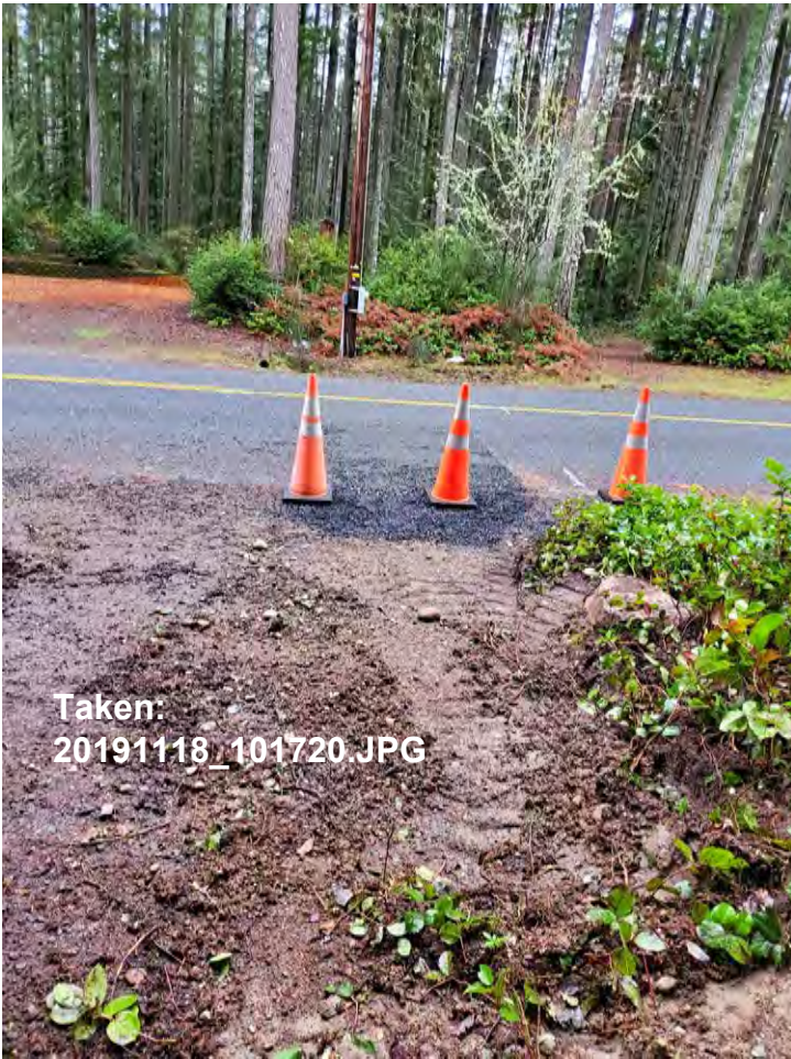
Taken: 20191118_101709.JPG Reference defining area of damage and markings
