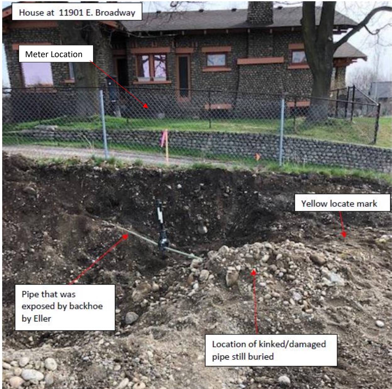
Attachment 4 – Picture of house at 11901 E. Broadway adjacent to the property that was being excavated. Location of damage.
