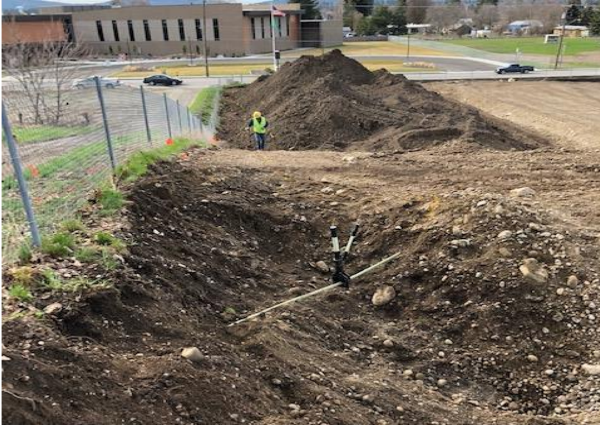
Attachment 7 – Looking south at damage and area being excavated.
