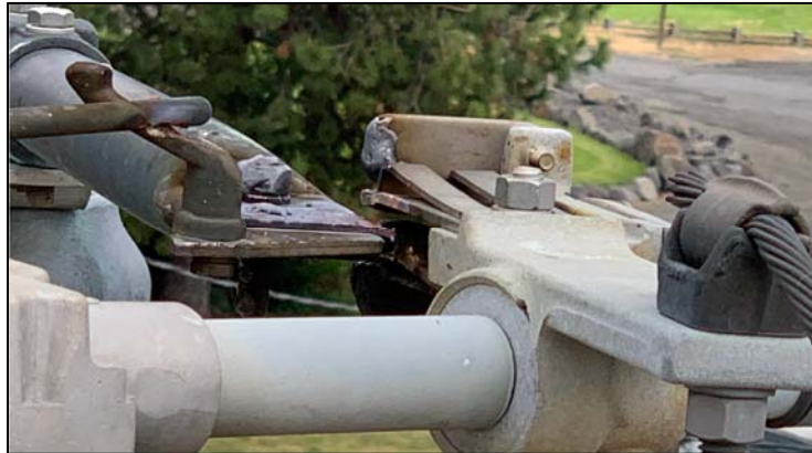
Figure 1. Damaged line switch
