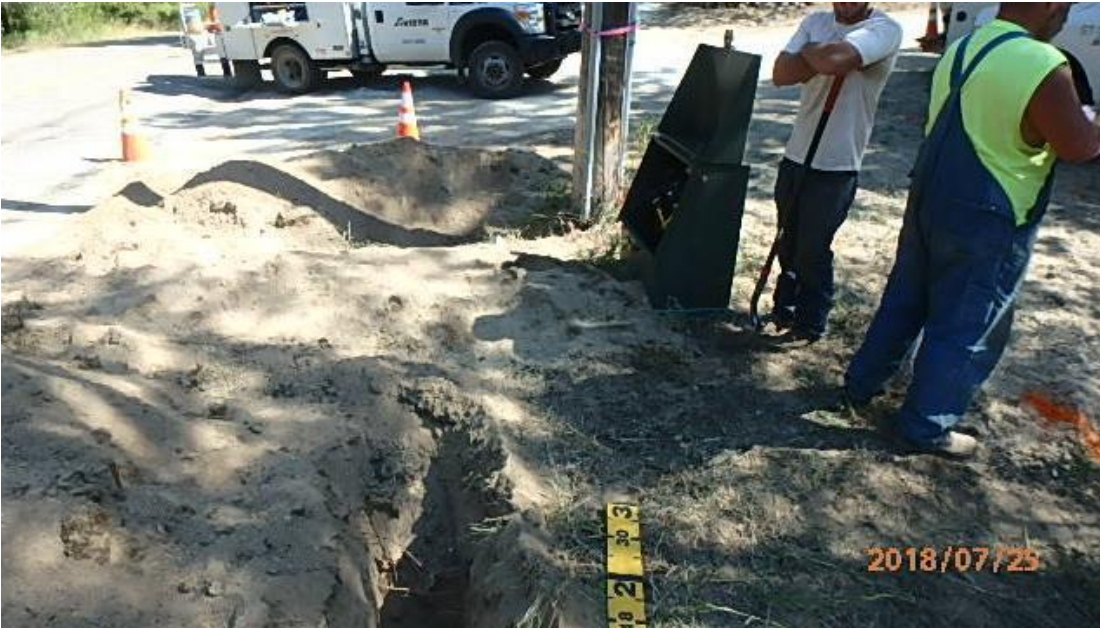
Attachment D: Pictures of damage location showing the pole and the date of the damage
