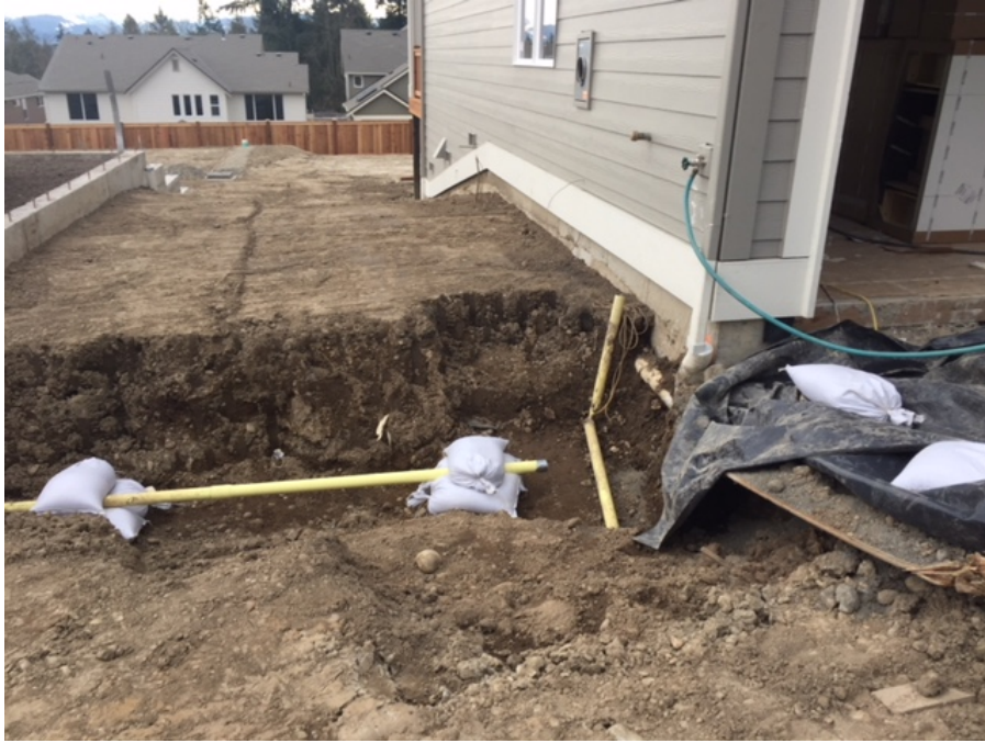
Evidence of Excavation without locates:
