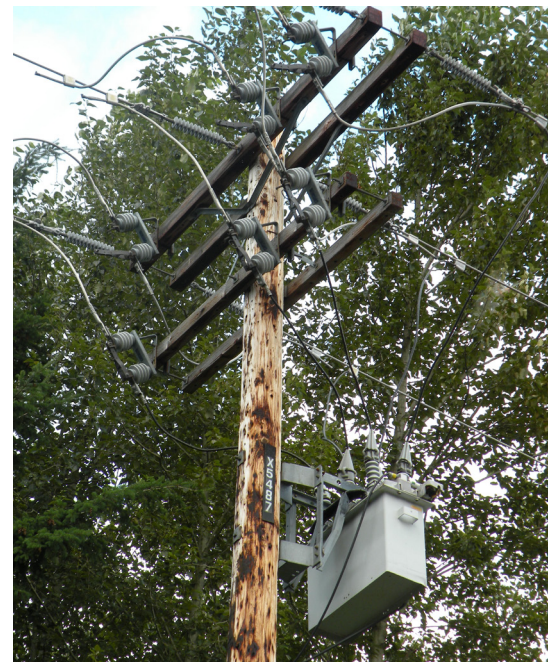
Recloser on PSE power pole
