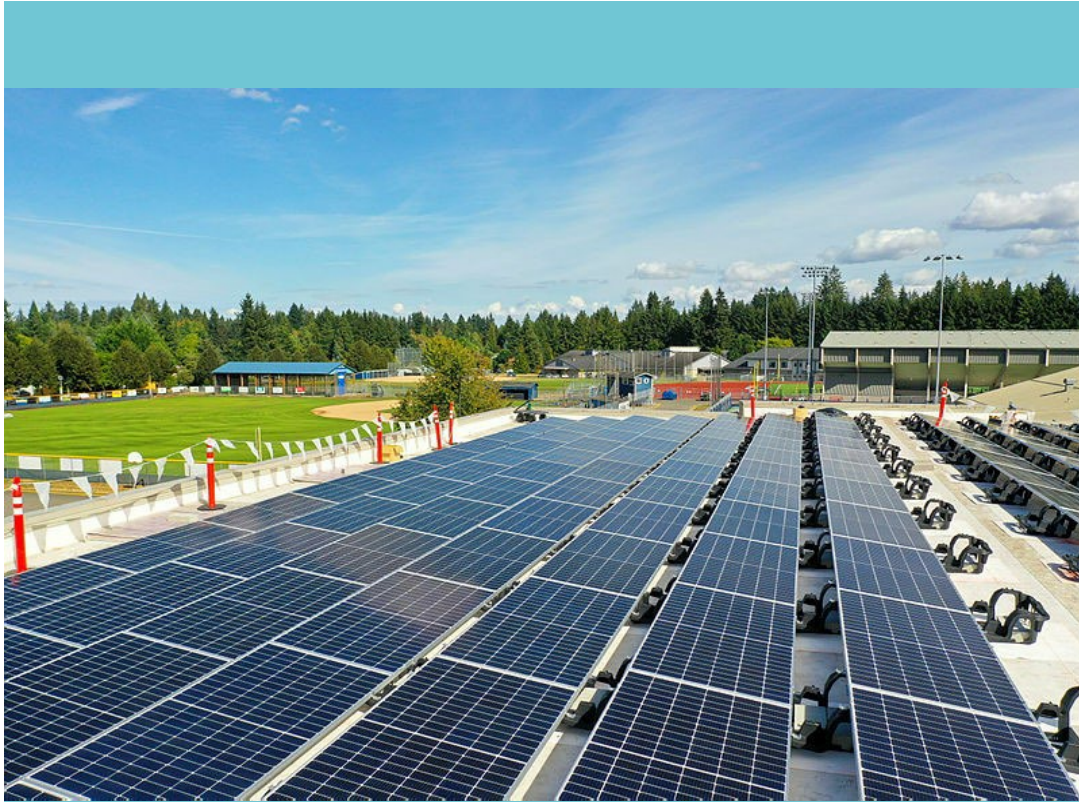
Community Solar Installation at Olympia High School
