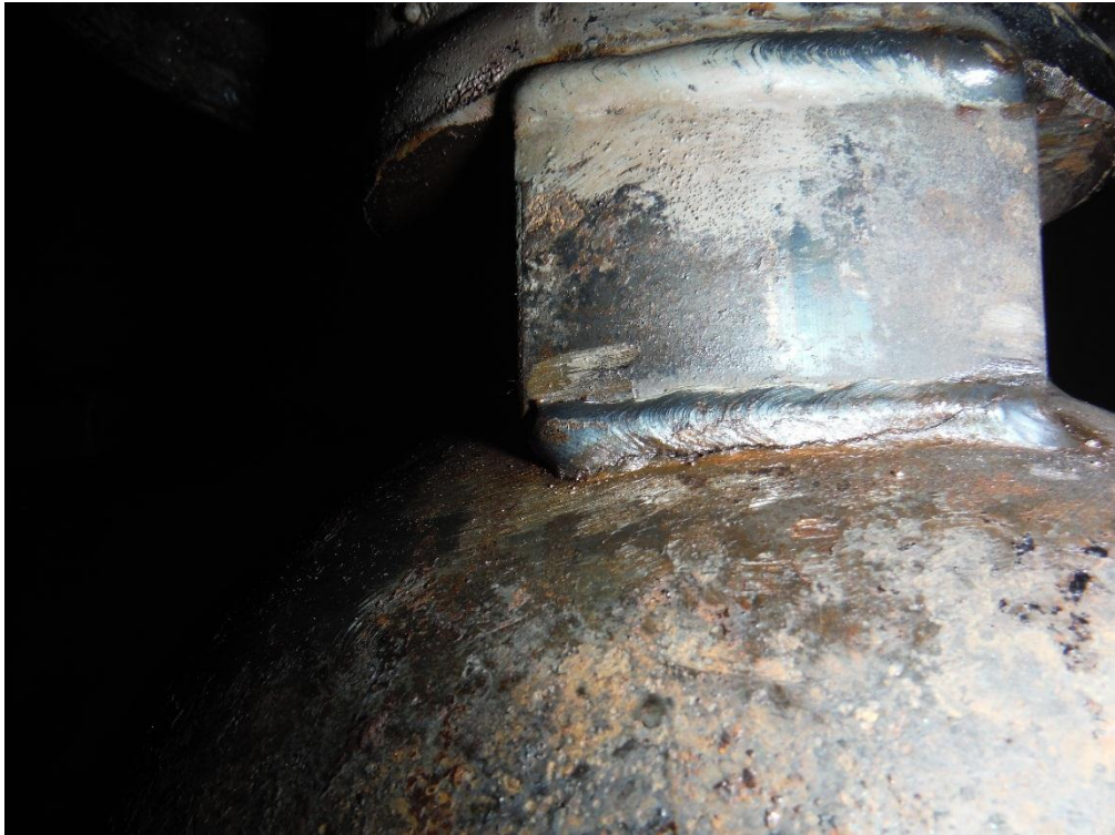
Stretch Duck axle with 2003 RTDI modification – possible cracked weld
