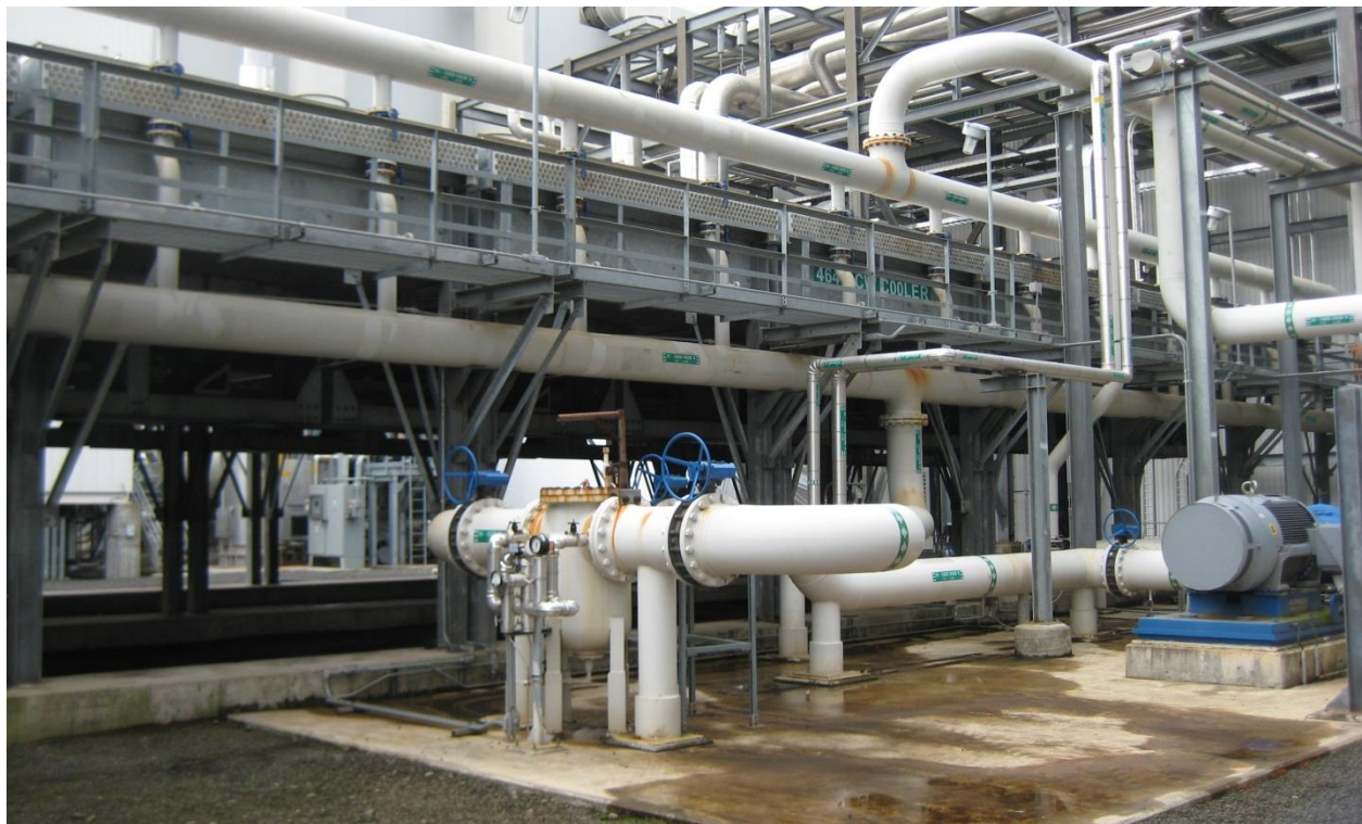
Figure 4: Closed cooling water system with cooler on the left and one of the two 550 HP pumps on the right
