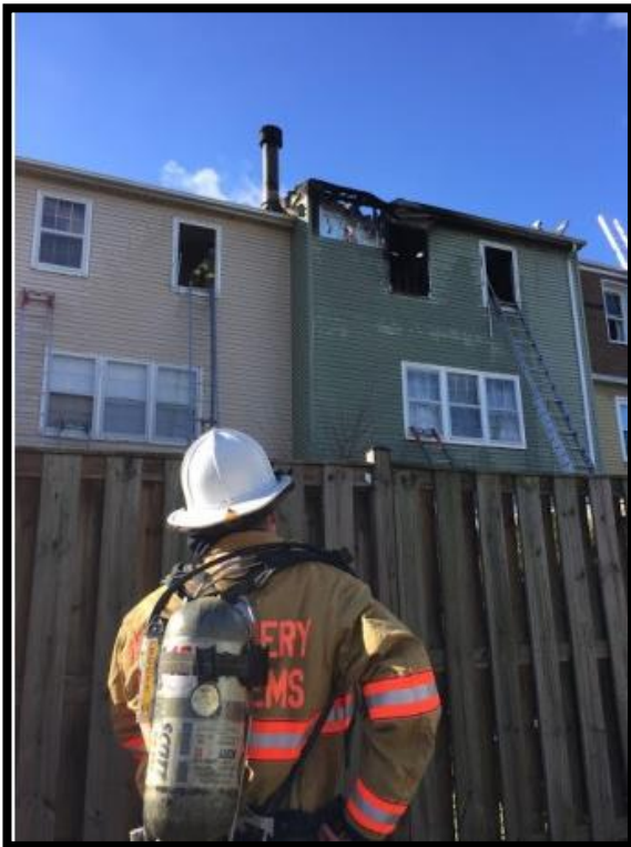
Aftermath of a space heater fire in Prince George's County, MD Source: http://patch.com/maryland/bowie/space-heaters-cause-bedroom-fires-twice-week-0
