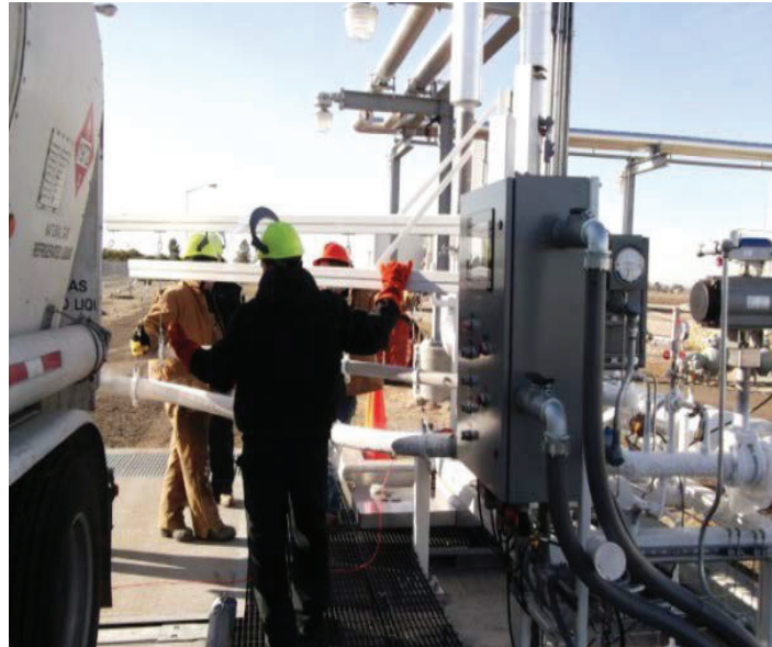
Figure 10 – Example LNG Truck Tanker Loading Operation
