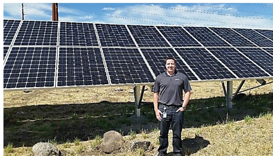
Left: Avista’s Community Solar Project
