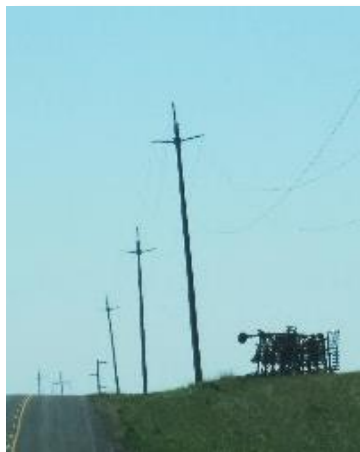
Ground inspection notes "leaners" on the Devils Gap – Line 115 kV Line
