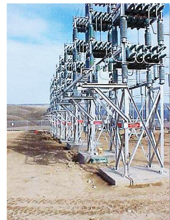
Dry Creek Capacitor Bank
