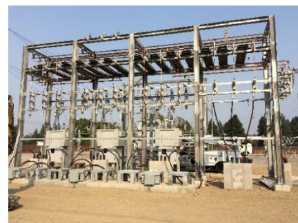
Ninth & Central Substation
