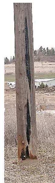
Ground inspection finds lightning-damaged pole
