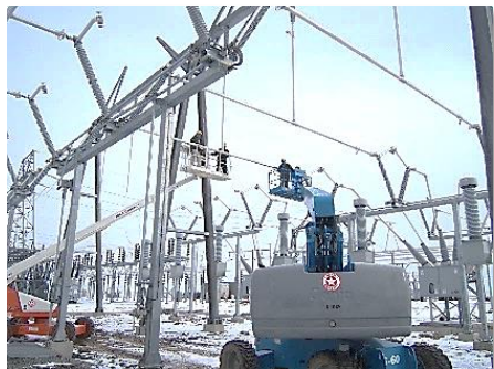
Building Benewah Sub
