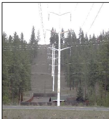
Bell-Westside 230 kV Line that Avista shares with BPA
