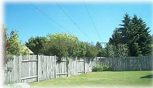
Backyard 115 kV transmission line with landscape trees directly underneath. Requires pruning every 2- 3 years.
