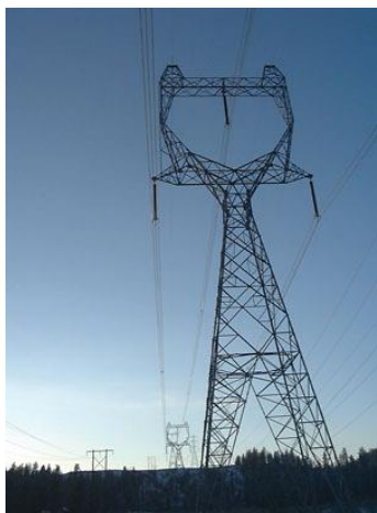
BPA's Bell-Coulee 500 kV line, built to help relieve congestion between Grand Coulee Dam and Spokane to the West Coast. (Avista's 230 line visible on the left.)
