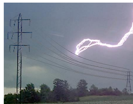
Lightning striking a shield wire
