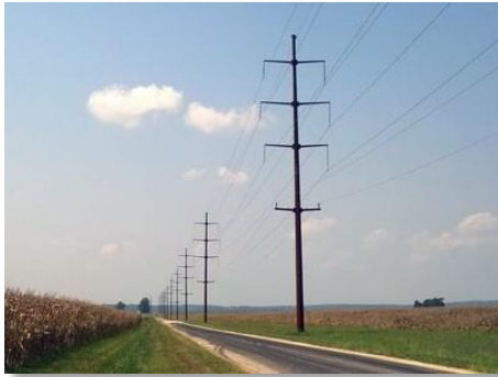
Transmission line (three arms above) with distribution underbuild below (single arm closest to the ground)
