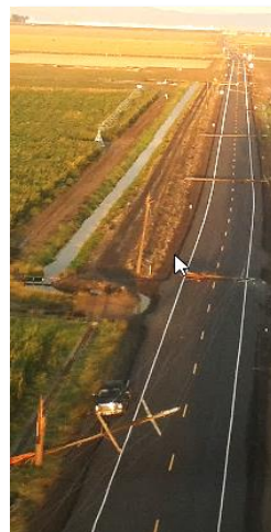
Right: Double Circuit Transmission Line (with ground wire on the top cross arms)
