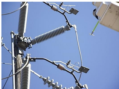
Installing air switches to help protect equipment and isolate faults
