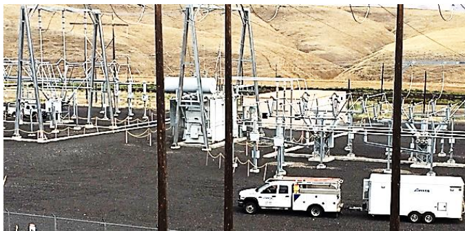
Dry Creek Substation
