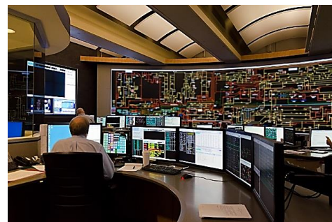
Typical Utility Dispatch Center
