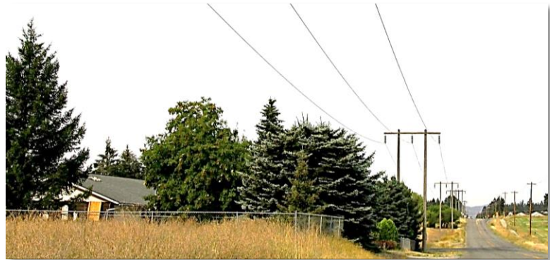
Roadside 115 kV transmission line. Requires aerial lift truck and chipper crew every 3 years to maintain clearance.
