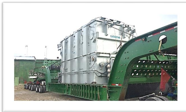
The new Pine Creek AutoTransformer
