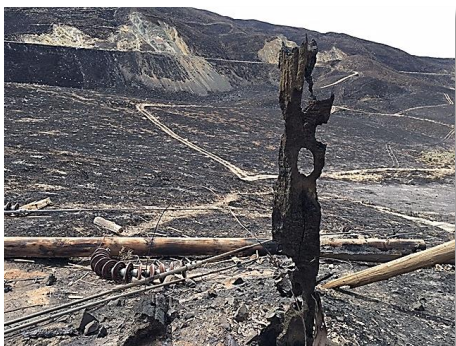
What is left of a transmission structure on the Walla Walla – Wanapum 230 kV line after a wildfire in August 2017.
