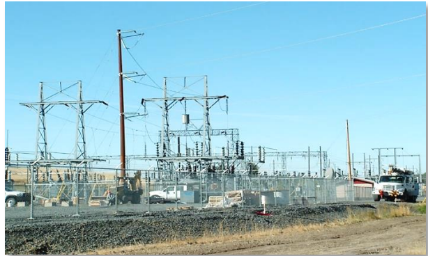
Typical Avista Transmission Substation
