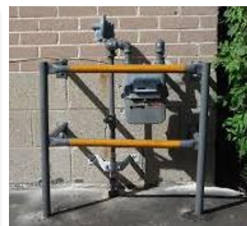
Gas Meter Barrier
