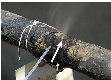
Gas Leak to be repaired
