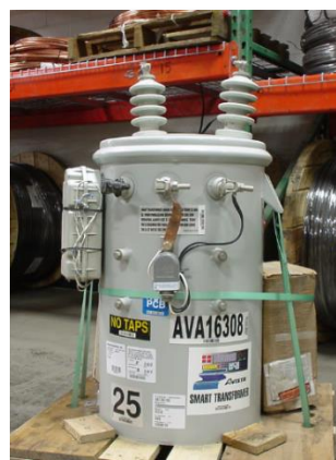
Left: “Smart” transformers provide the exact amount of power needed, respond to fluctuations and act as a voltage regulator
