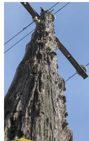
Some of the Avista Distribution poles installed in the 1920's and 1930's are still in service today... and it shows!
