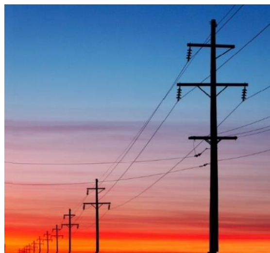
Transmission Poles showing distribution lines “underbuilt” below the transmission lines, which puts additional strain and wear on the poles
