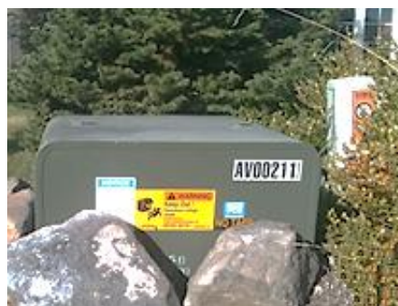
Left: Landscaping features block Avista access to equipment
