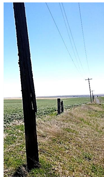
Split Pole – old stub in background
