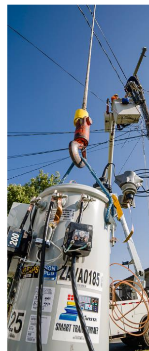
Avista “Smart” Transformer
