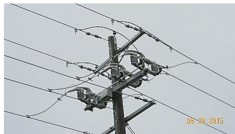
Above: Spokane Smart Grid Switching Device
