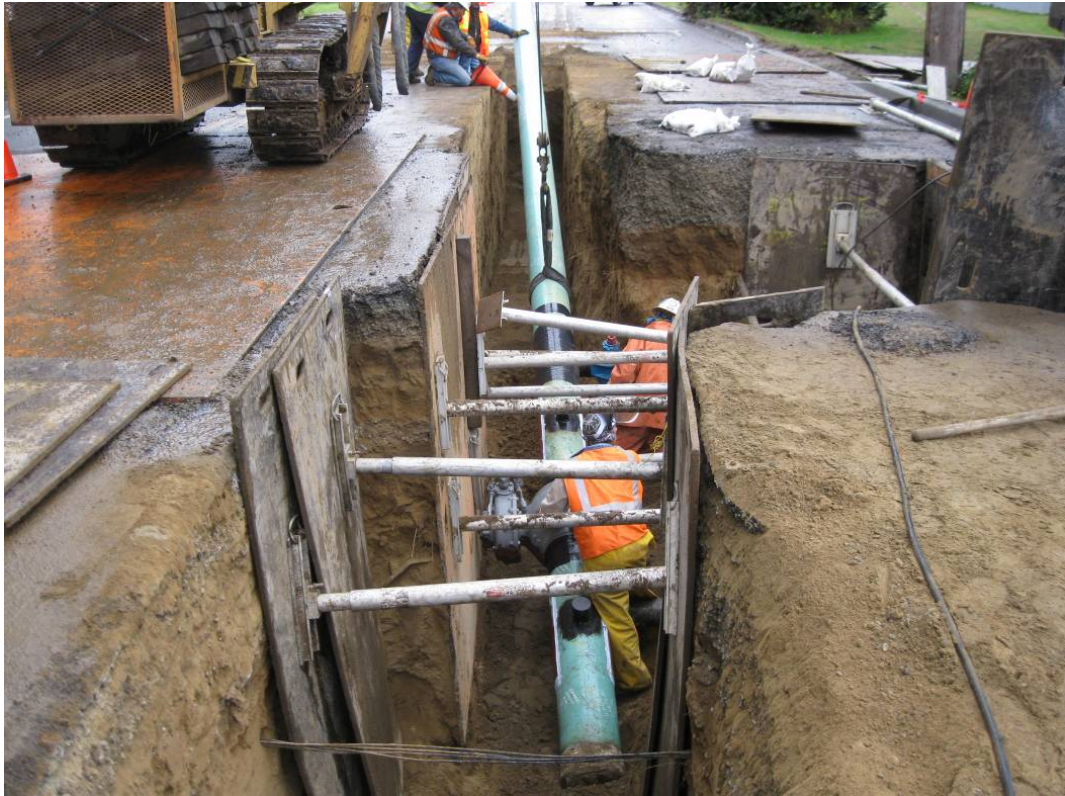
Figure 4-6: Lacey-Fones Road, 12-Inch Diameter Supply Pipeline, In-Service 2009
